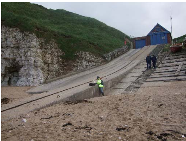
Lifeboat Station, slipway and revetment at North Landing (Asset Ref No. 1231D901D3201C02)
