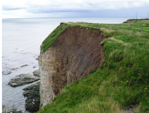
E111/14 erosion of the till cap near Stottle Bank Nook (Partly Active)
